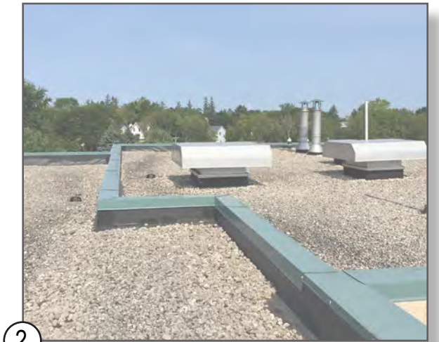
② ROOFTOP VENTS
