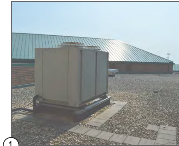
① ROOFTOP MECHANICAL UNIT
