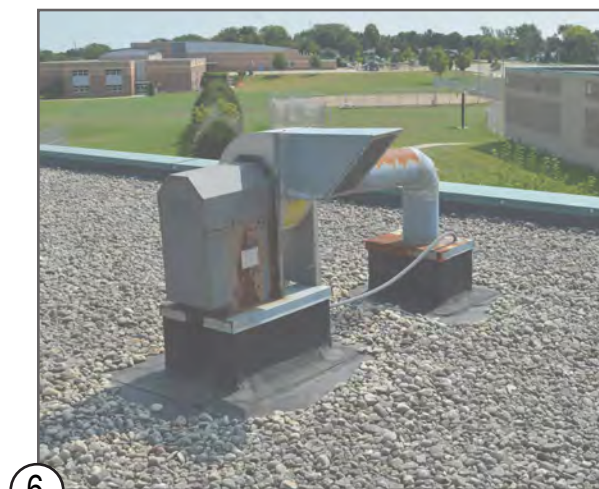
⑥ ROOFTOP MECHANICAL EQUIPMENT
