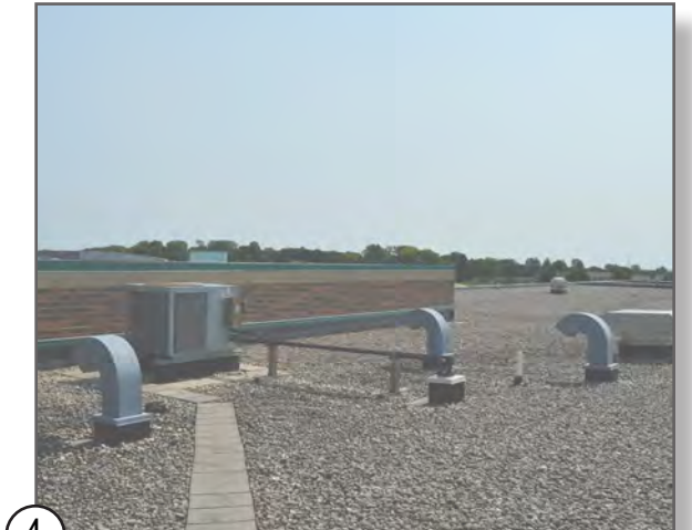
④ ROOFTOP MECHANICAL UNIT & VENTS
